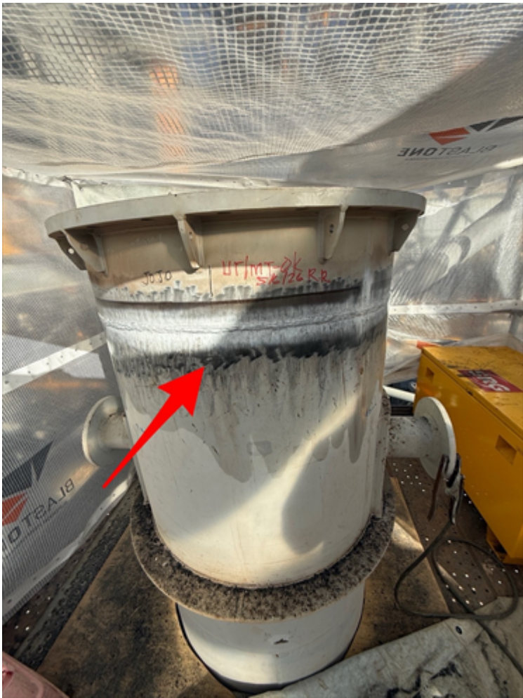
Drawing / ISO No: C14-005-MEC-DRG-002; Spool No: Flange; Weld No: W1; Welder ID: 076/080/086; WPS No: 283; Welding Process: GTAW/MMAW
